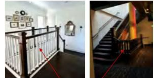
Guardrail at open floor must have bracing within the floor
